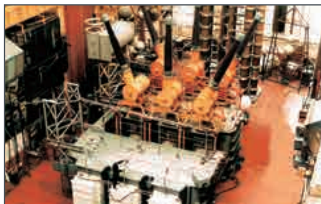
Figure A4.11: Large transformer
