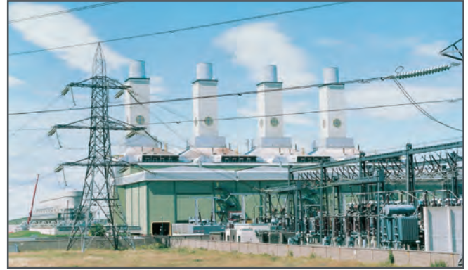
Figure A1.1: Power station
